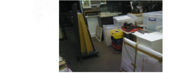
Fig. 6. Unlagged or poorly lagged hot water heating pipes were discovered running under the entire length of the floor of this art store during a recent energy conservation survey. They ran right under a large permanent area of clutter where the temperature of the carpet was at 23°C, making this area under the boxes and tables ripe for a pest infestation.
